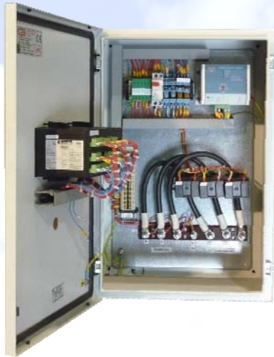
The command and control panel (the TCGE)
